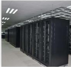
Computer room monitoring
