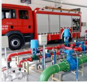
Fire Control System
